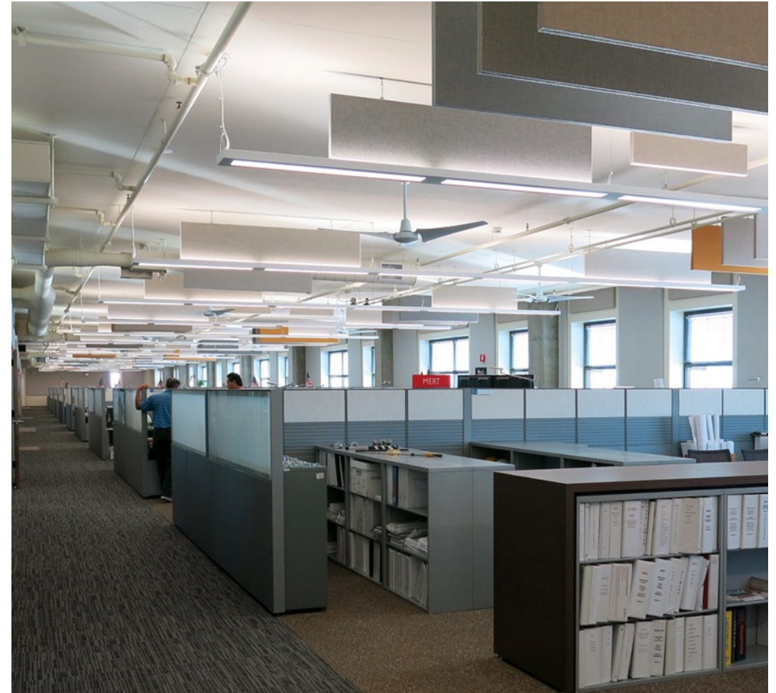
SMUD East Campus Operations Center has radiant and ceiling fan system
