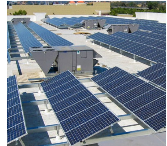
Rooftop mounted PV
